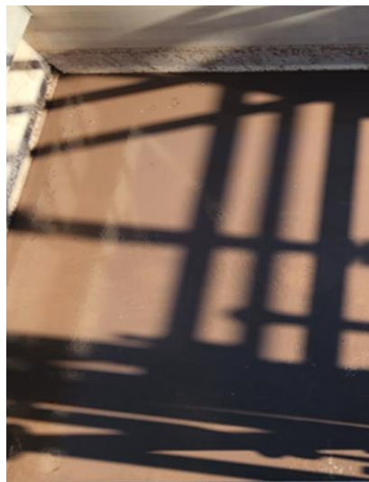
Fig. 4. Muddy surface of Opal's SWTP Clarifier due to the filamentous bulking @ 203 mL/g SVI30.
